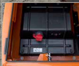
Battery cut-off switch
